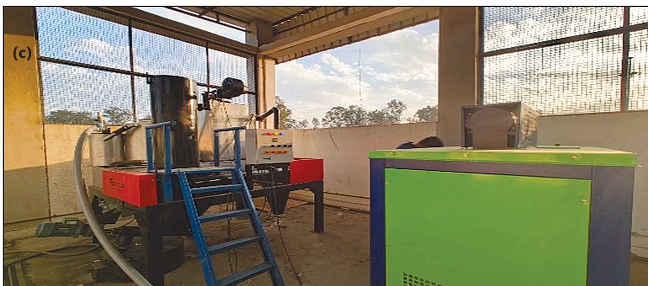
a) Biomass Pellet Machine; b) Portable Gas Analyzer; c) 10KVA downdraft agro-residue gasifier
